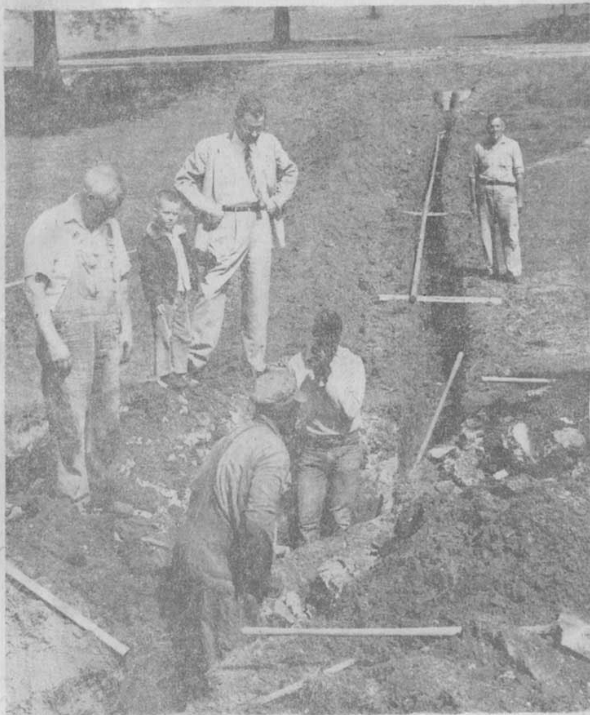
NEW WATER SYSTEM —Bonny Oaks School is getting a new water system. Brainerd Water Works is installing the system for them and water from this organization will be used by the school. The old school water system will be used by the school laundry and the school barns. Shown watching the work are, left to right, H. T. Smith, maintenance superintendent for the county; Michael Adamson, 5; Malcolm Adamson, Bonny Oaks superintendent, and Ed Boriz, county plumbing and heating superintendent.
